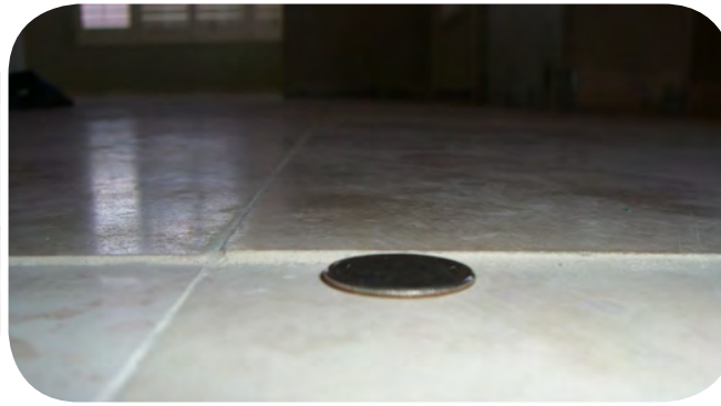
LIPPAGE (UNEVEN TILES)
