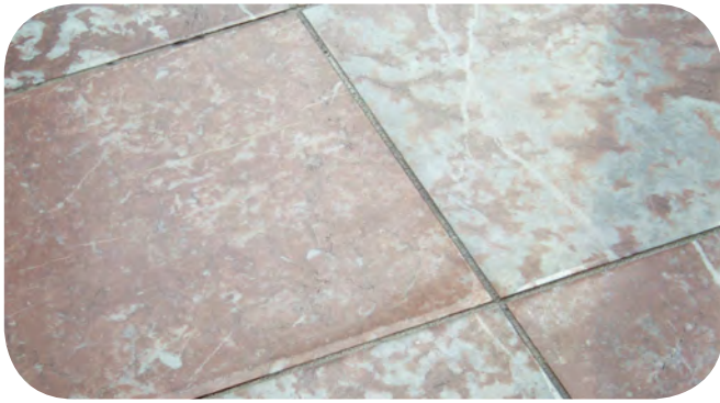
DIRTY, STAINED GROUT LINES
